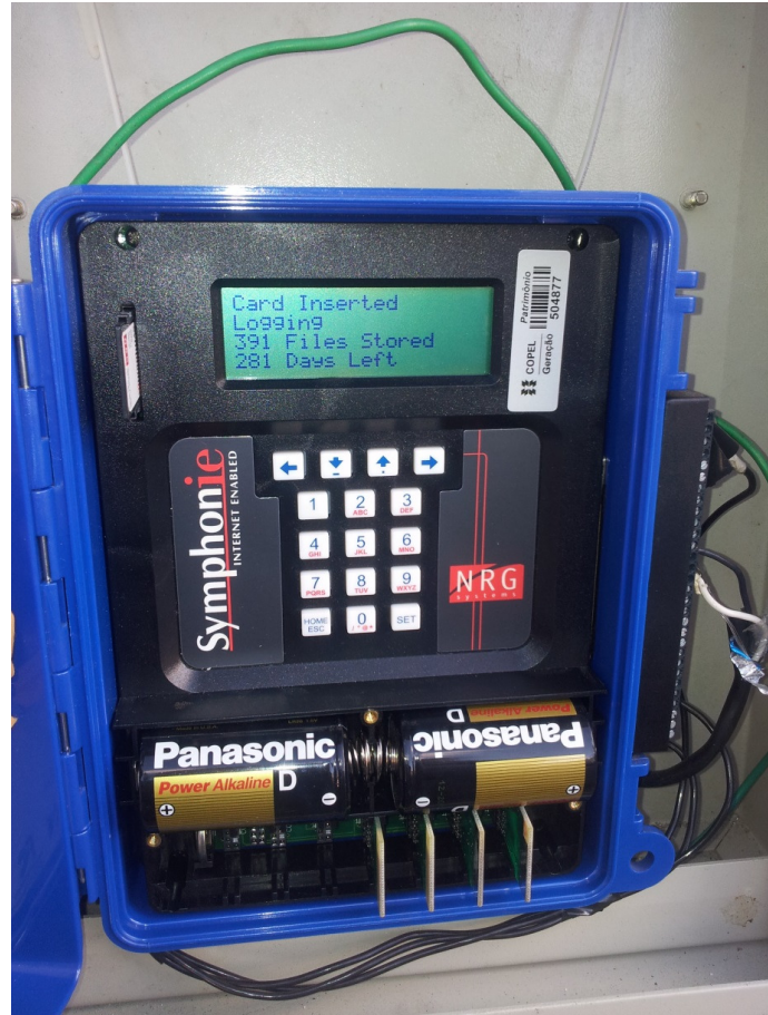
Figura 9: Data logger instalado na UTFPR.
