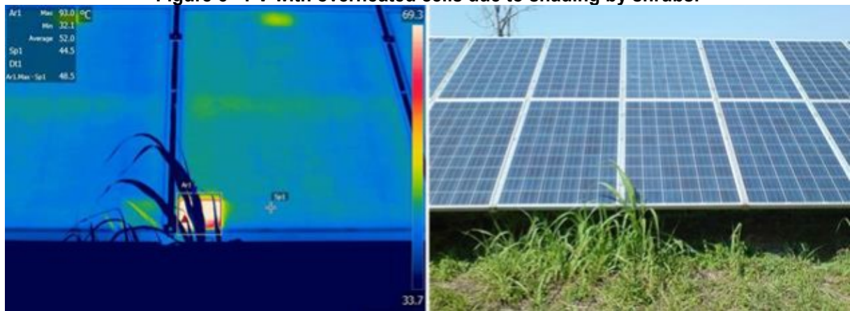
Figure 6 - PV with overheated cells due to shading by shrubs.
