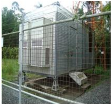
Figura 5 - ERB Greenfield Indoor (container)
