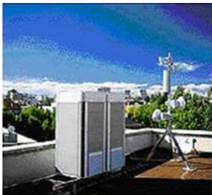
Figura 4 - ERB Roof Top Outdoor
