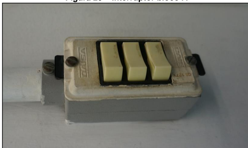
Figura 29 – Interruptor bloco A
